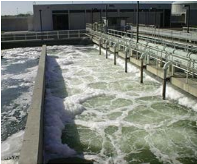
Image No. 31: Aeration basins.
